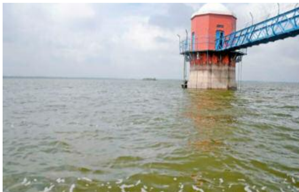
The project would also include works on strengthening the bund and repairing sluice gates of these reservoirs
